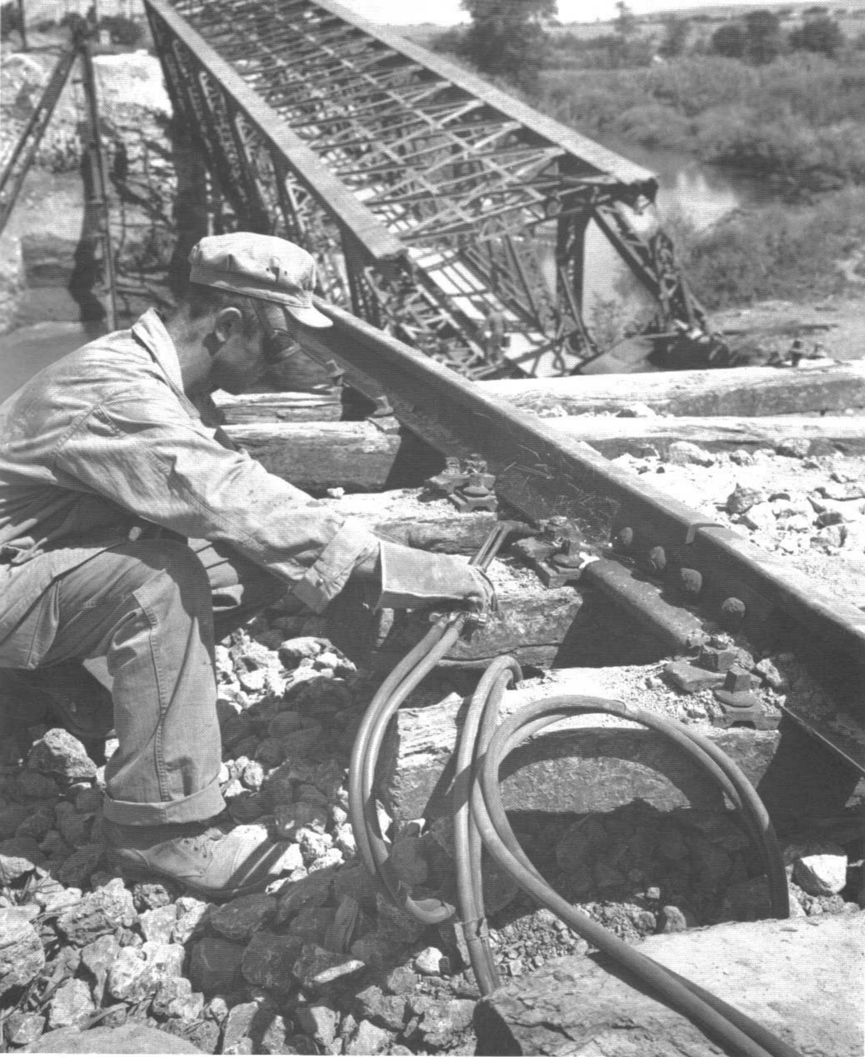
A U.S. Army welder cutting rails which were wrecked in bombing at the Malta River bridge near Civitavecchia, Italy. (7-20-44)
