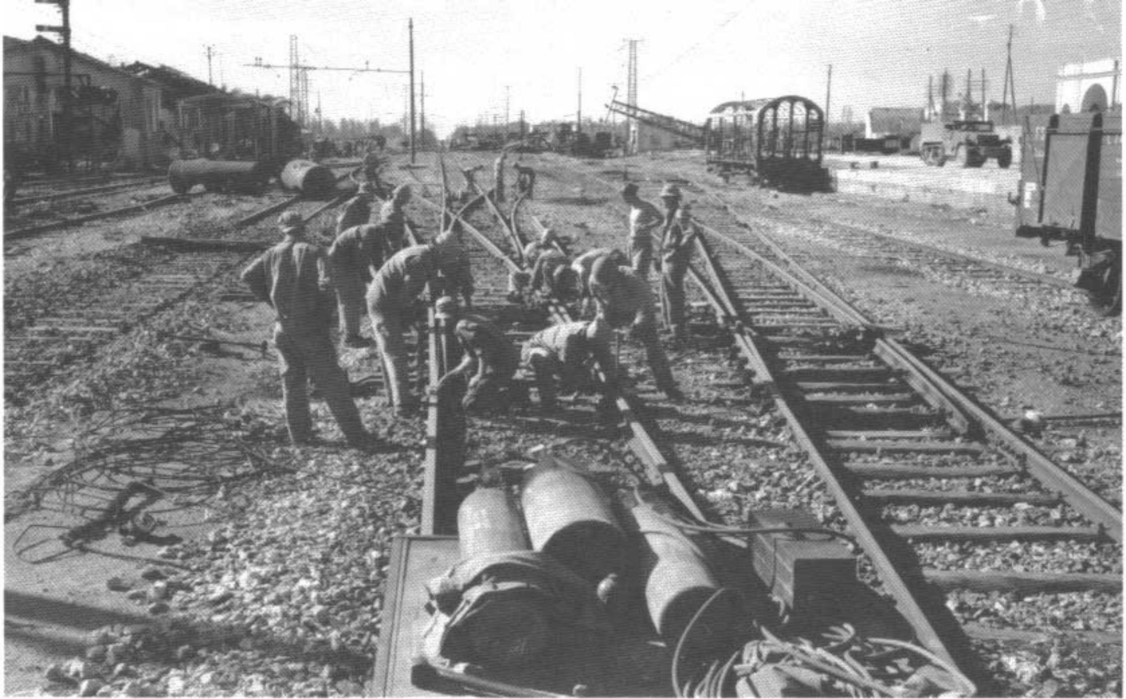
Engineers repair the railroad station in Caserta, Italy. Its rails had been blown up by the Germans at 100 foot intervals. (11-6-43)
