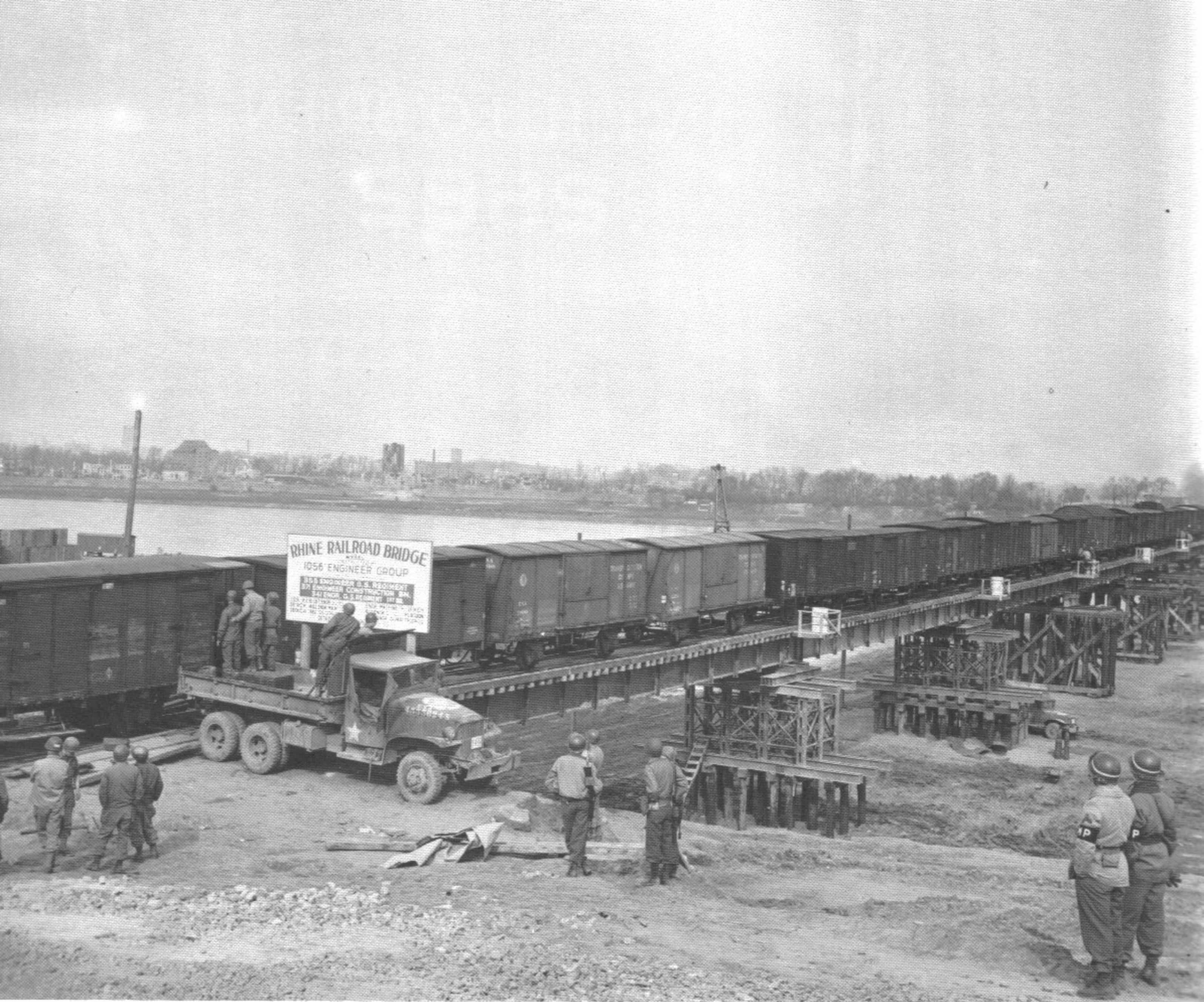
Supply trains roll across the Robert Gouldin railway bridge over the Rhine River. The engineers of the Advance Section Communication Zone completed the bridge and approaches in 10 days. (4-10-45)
