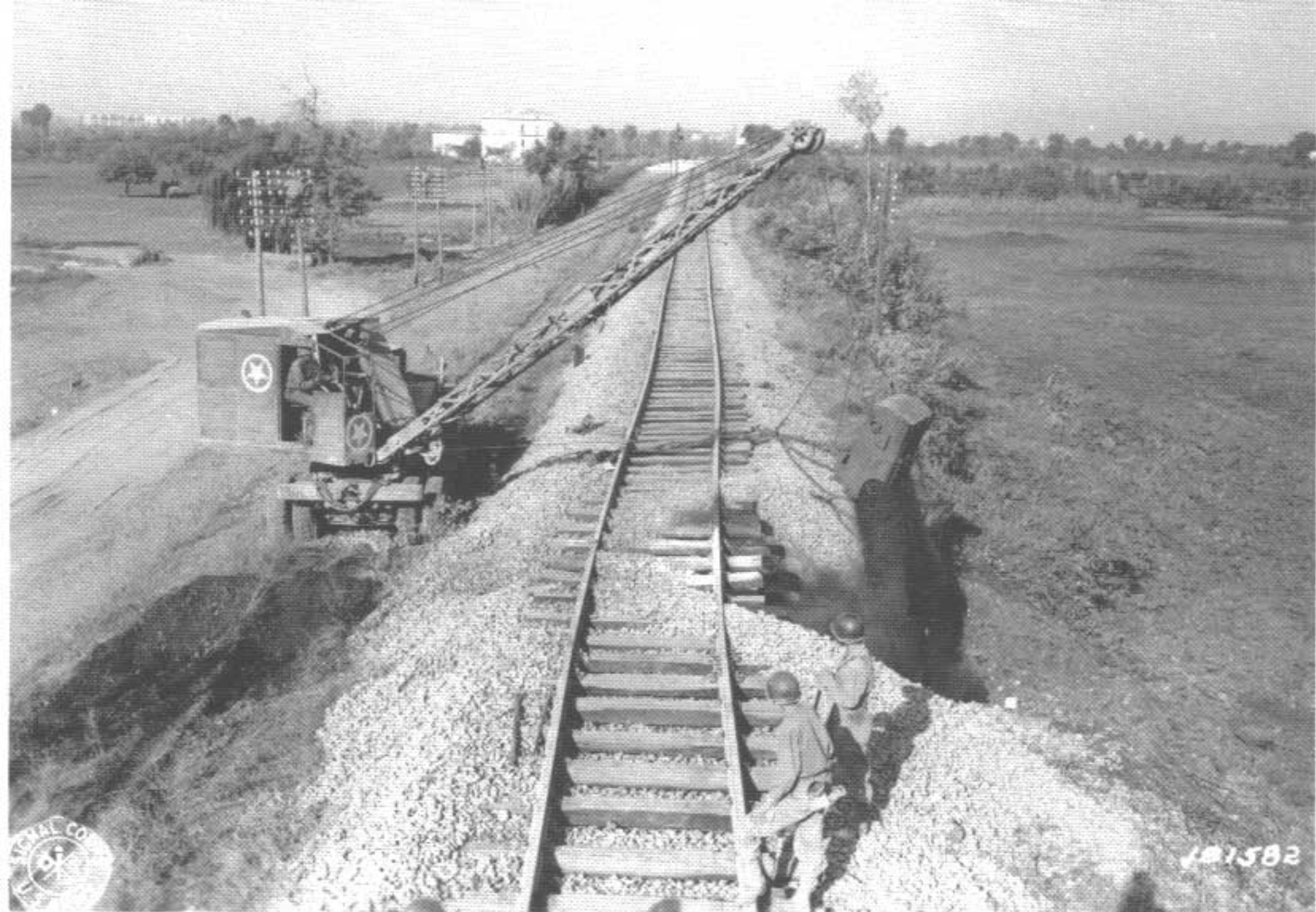
The 36th Combat Engineers use a crane to fill a crater before straightening the tracks near Battipaglia, Italy. (9-26-43)
