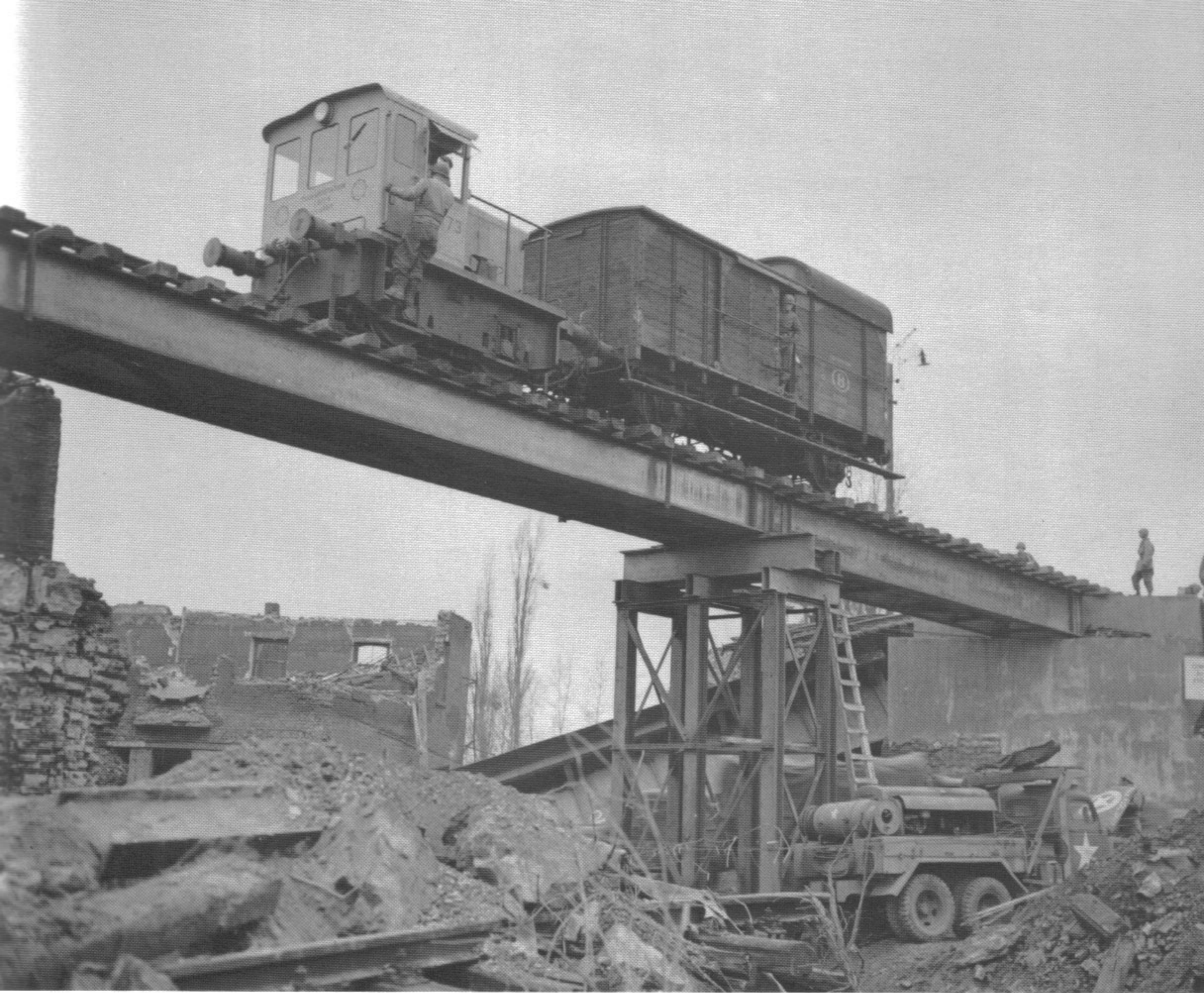
Destroyed by the retreating Germans, this new bridge was built by the 33rd Engineers of the 30th Division. (12-16-44)
