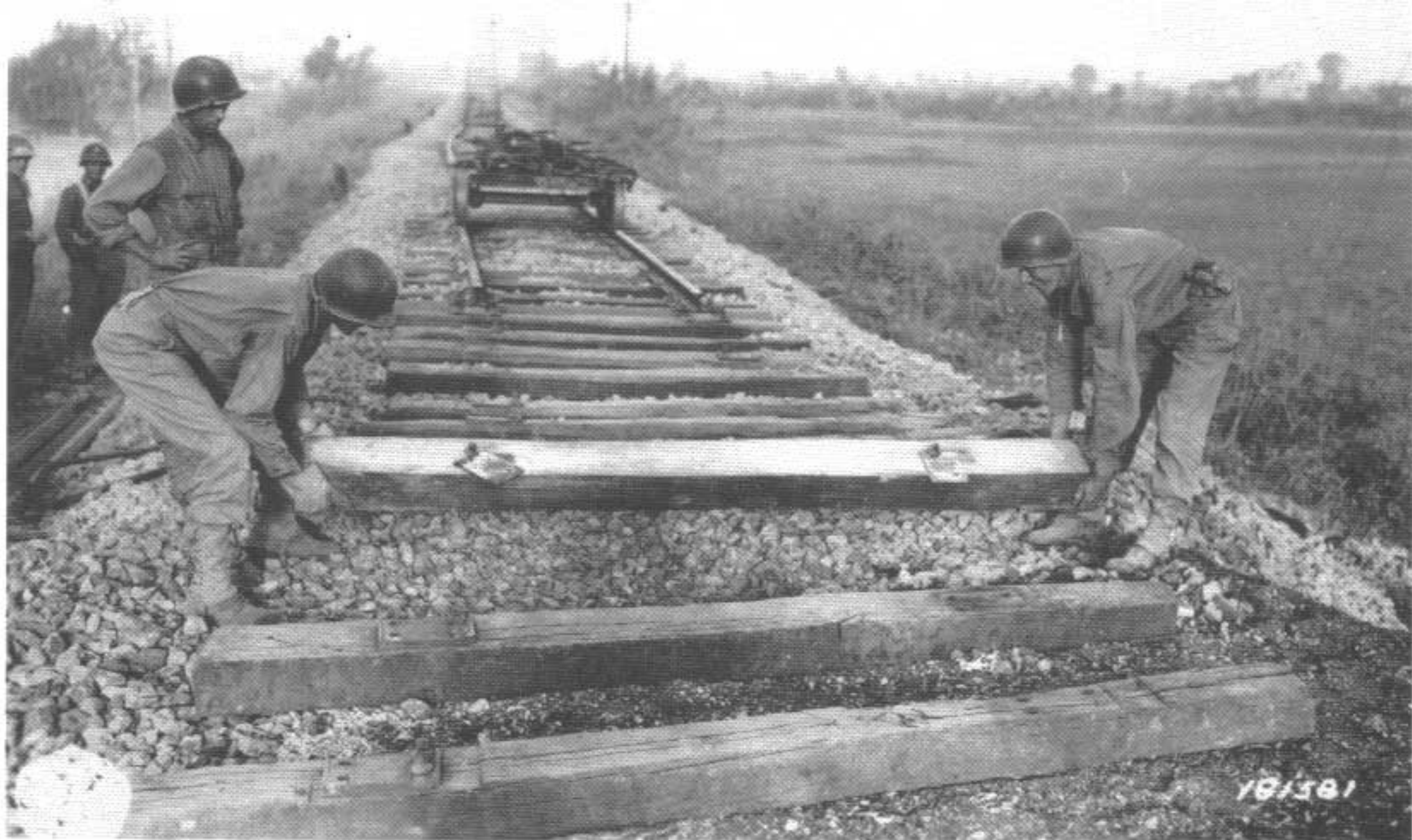
Pvt. Lewis Hinaman, Bine Meadow, CN, and T/5 Lauri Arklander, Andover, OH, 36th Combat Engineers, replace a tie near Battipaglia, Italy. (9-26-43)
