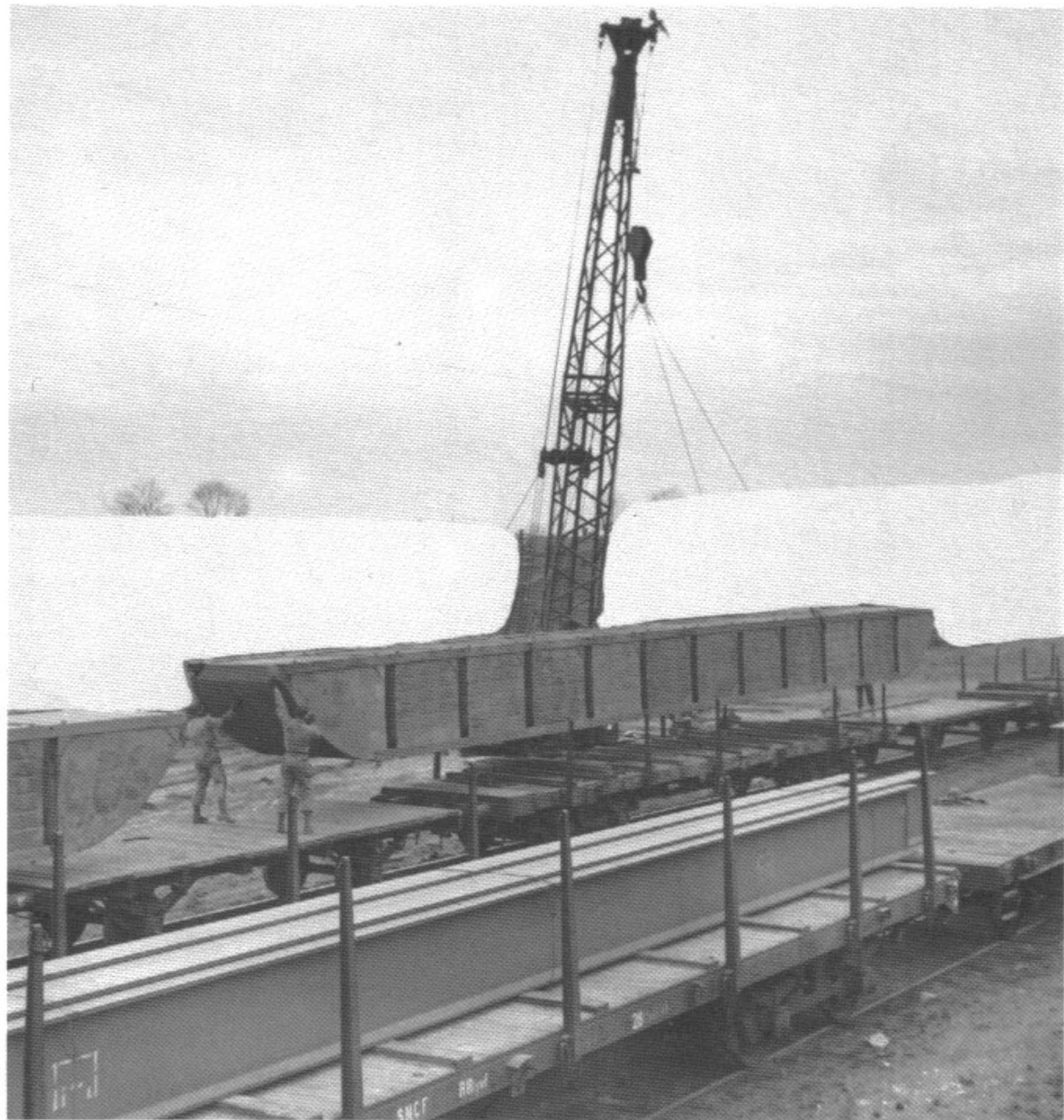
A string of Navy pontoons, guided by U.S. Army Engineers being lowered onto flat cars by a Lorain 82-30 ton lift crane, were used in the construction of the "Lincoln on the Hudson" railway bridge across the Rhine River, Germany. The background was obliterated by military censors. (3-25-45)
