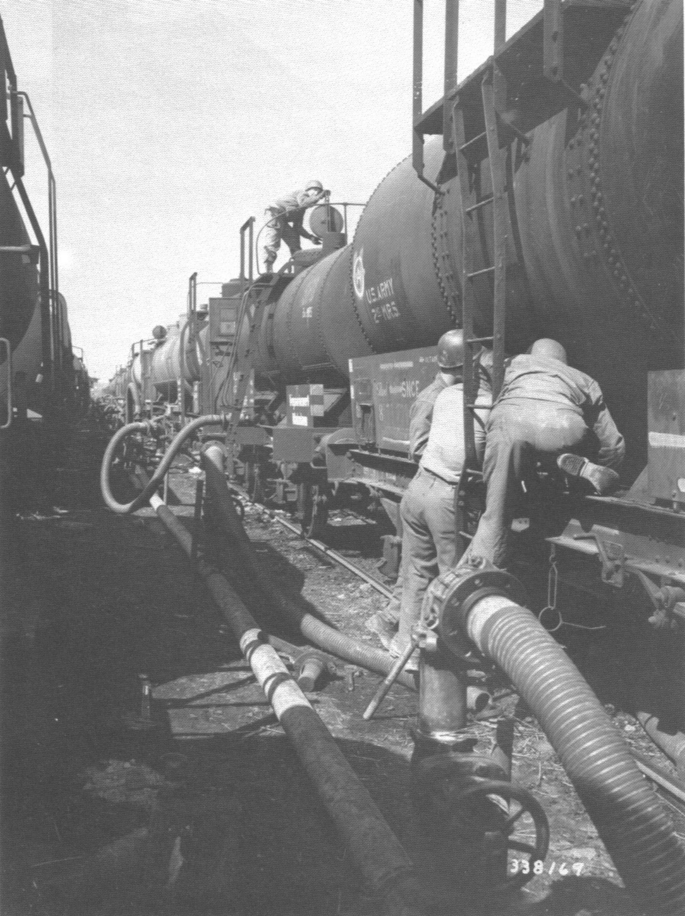
G.I.'s repairing a leaky valve on an old German tank in the Mehlen, Germany, railroad yards. The tank cars unloaded their gasoline into storage tanks through a pipeline across the Rhine, from which the gasoline fueled the 1st Army drive into Germany. (4-9-45)
